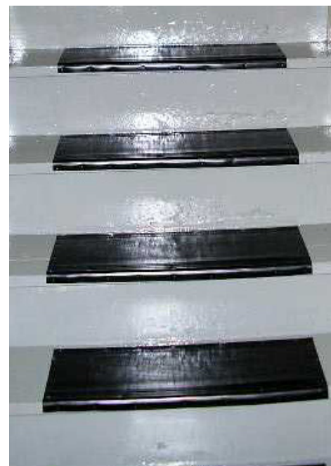
FIGURE 5.6b Friction hazard on stairs post-treatment.
