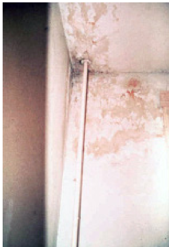
FIGURE 13.2 Deteriorated paint on surfaces that are unsuitable for encapsulation
