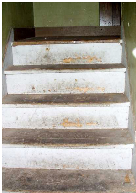
FIGURE 5.6a Friction hazard on stairs pre-treatment.
