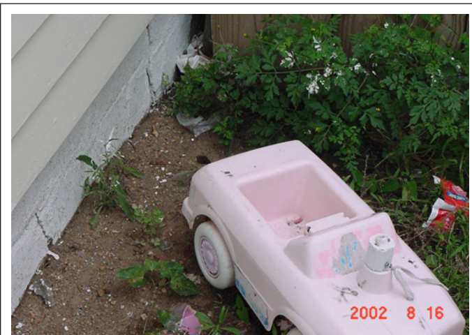
FIGURE 5.9 Soil lead hazard at dripline
