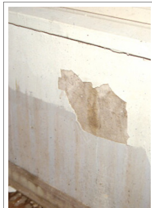
FIGURE 5.5 Baseboard showing a de minimis amount of deteriorated paint.
