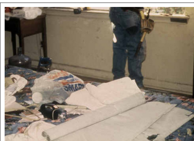
FIGURE 4.3 This worksite was not properly prepared for lead-disturbing work by removing the occupant's belongings.
