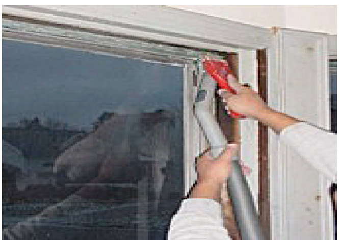
FIGURE 11.12 Vacuum window again.
